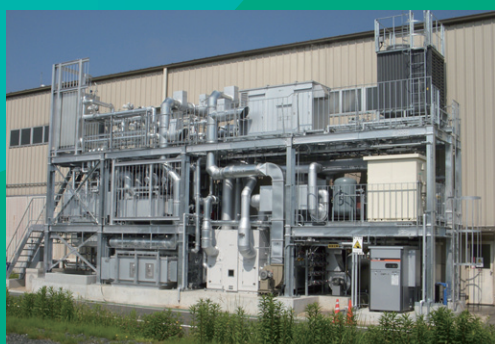
Cogeneration equipment at Ibaraki factory
